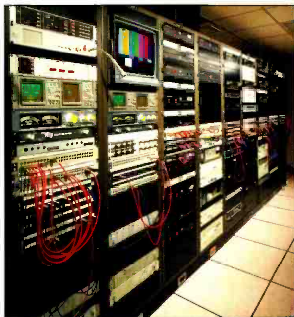
Atlantic Satellite is linked by 50 digital fiber lines to Waterfront facilities, and the uplink service utilizes Waterfront for delivery of video. Atlantic Satellite's satellite receiver rack is shown here.
