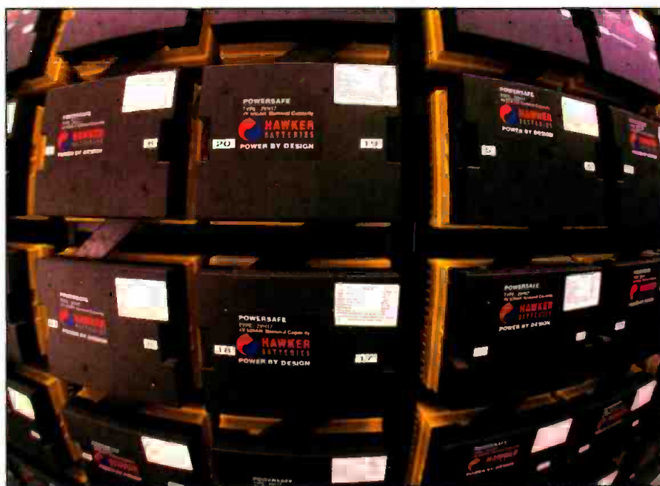
The amount of backup time available to a facility depends on the power available from its battery bank. Shown above is a section of the available batteries at the International Broadcasting Center at the Sydney Olympics. (See page 94.) Photo courtesy Telstra.
