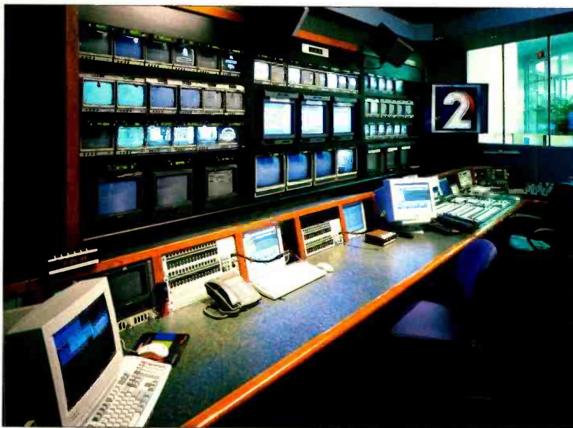
Master Control at KHON-TV in Honolulu, HI, on the air in 1999. Photo courtesy Digital Systems Technology.
