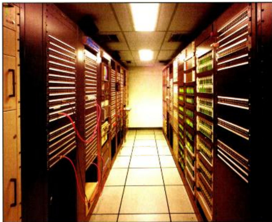
Waterfront's router support wiring rack room.
